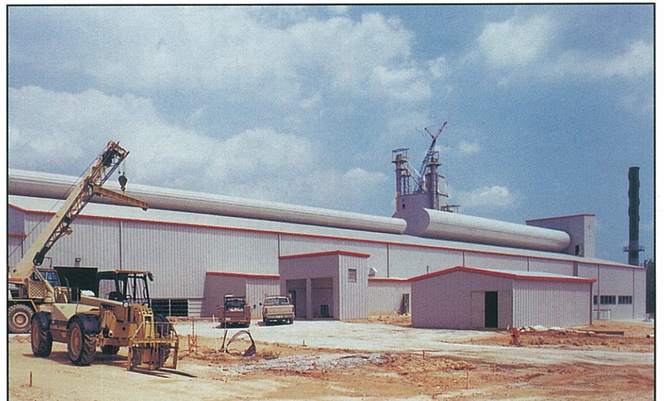
One of Span Construction & Engineering's many projects from the past year was the Cardinal Float Glass Plant in Mooresville, NC. The facility measures 450,000 sq. ft.
