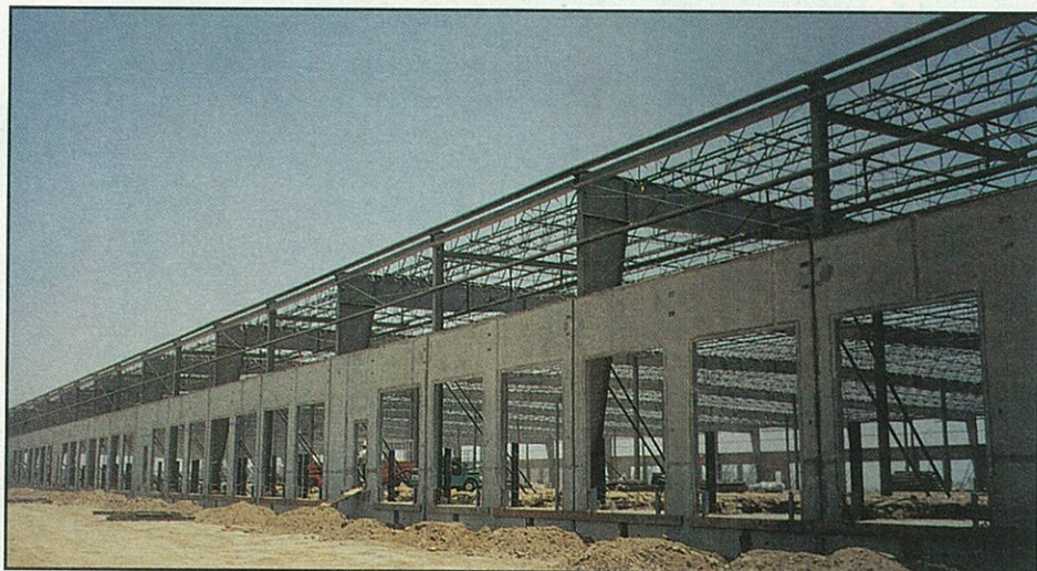
Located in Mira Loma, CA, the Costco Distribution Depot was a 900,000 sq. ft. project.
