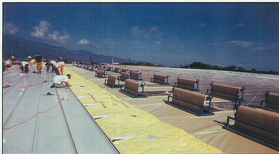
The insulation is installed on the 135,000 sq. ft. Costco Wholesale building in Maui, HI.
