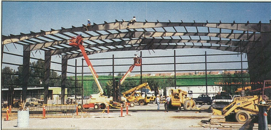
This 24,000 sq. ft. transfer station for Browning-Ferris Industries, Fresno, CA, was among Span Construction's 1993 accomplishments.
